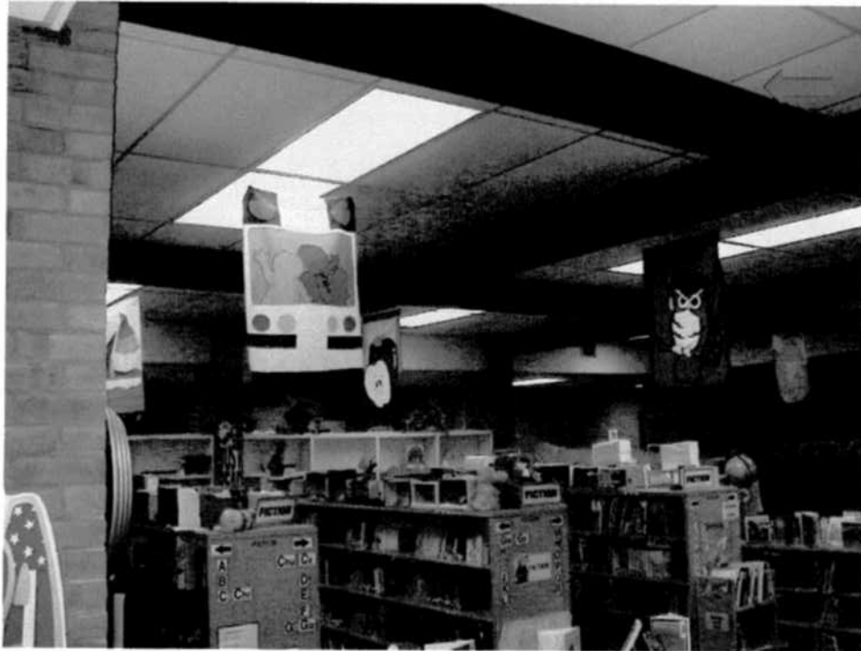
Photo 10: Horizontal cracks in wood framing over library.
