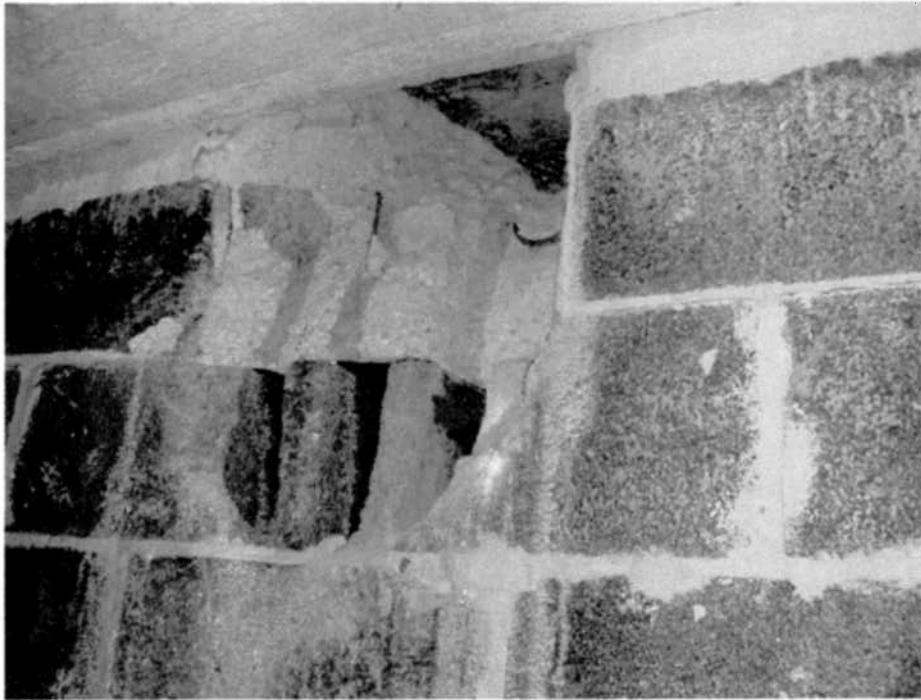
Photo 6: Wall damage at addition tie-in.
