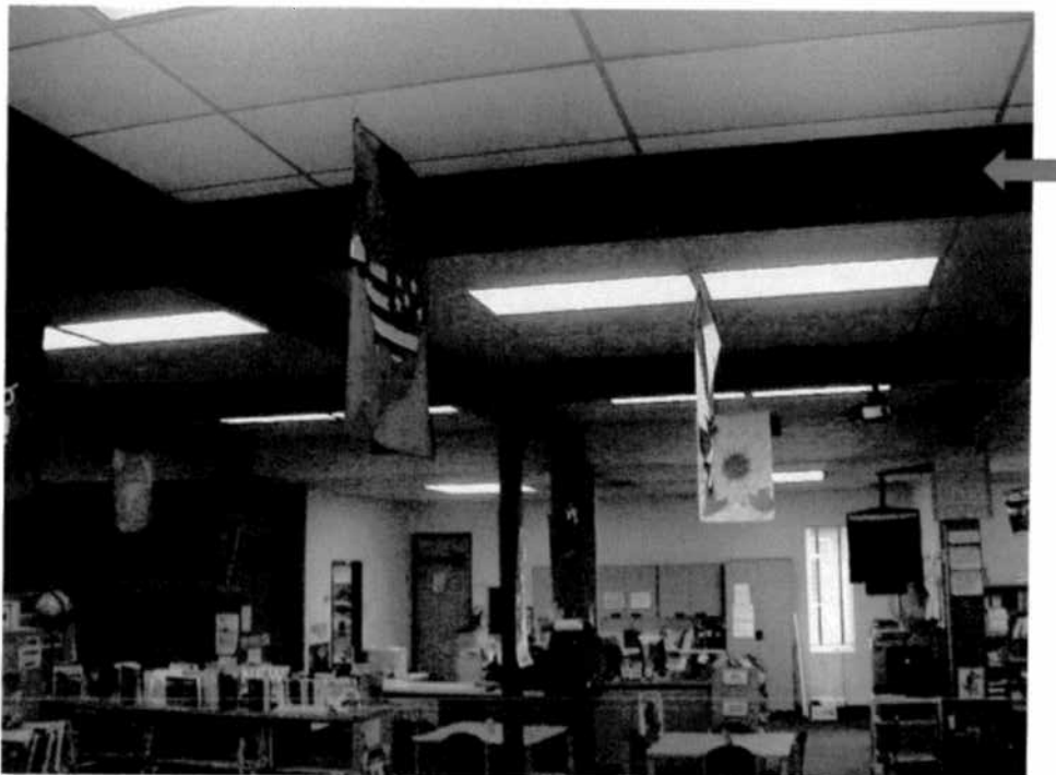
Photo 11: Roof framing with horizontal cracks.
