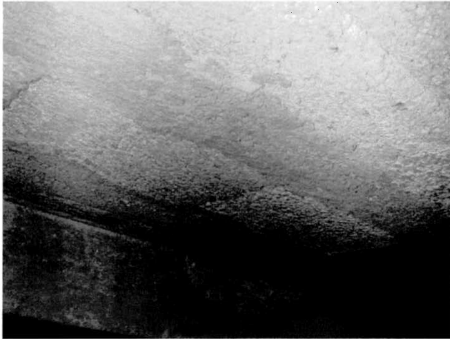
Photo 4: Notched concrete beam.
